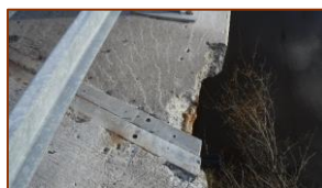
Full Depth Spall at Deck End
