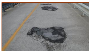
Asphalt Patched Spalls in Deck
