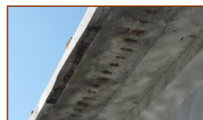
Spalling and Delamination in Soffit
