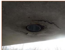
Delamination at Southwest Deck Drain
