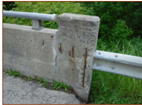
Spalls in Barrier Wall
