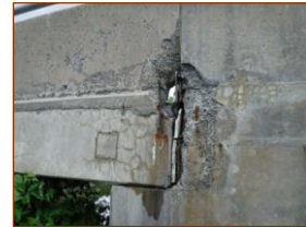
Spalling at Joint Exterior at Southwest
