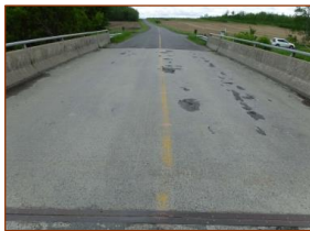
Asphalt Patched Spalls in Deck
